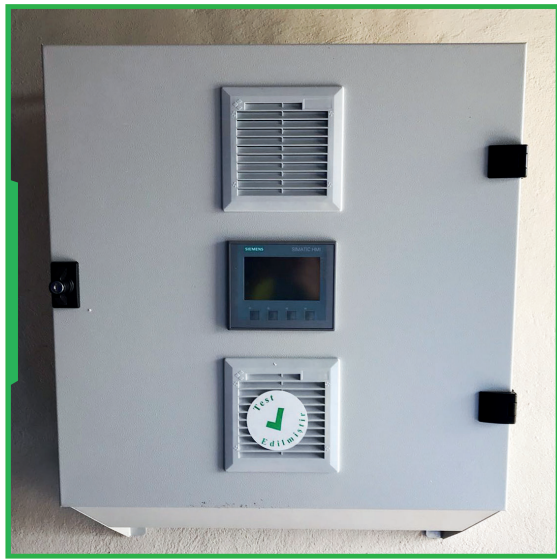
Alarm Control Unit (ACU)
